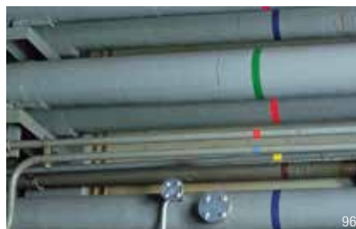
For colour-coding pipes with 3M™ Vinyl Tapes, select from either nine vivid colours or transparent to let underlying colour show through. Backing is coloured throughout to help maintain ready visibility.
